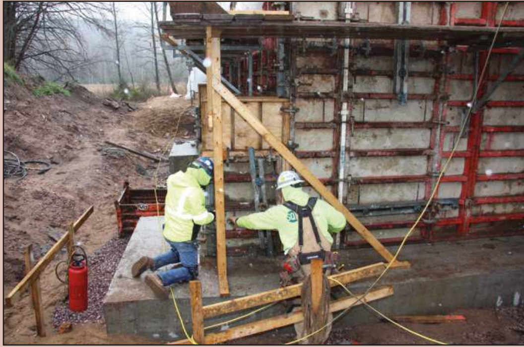
ON THE JOB at the Marquette Wastewater Treatment Plant expansion are cement finisher Tim Etter of Bricklayers and Allied Craftworkers Local 2, with Robert Locke of Laborers Local 1146, employed by Miron Construction.
