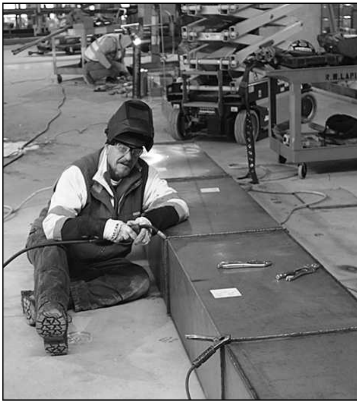
SHEET METAL WORKERS Local 7's Trevor Smith readies a weld on a grease duct set to go in a kitchen area at the Gun Lake Casino Hotel project. He's employed by R.W. LaPine.
