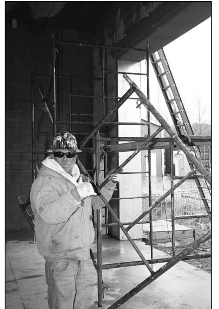
AT WORK AT THE Marquette Wastewater Treatment Plant project is Jack Lambert of Bricklayers and Allied Craftworkers Local 2. He's employed by John Buckland Construction.
