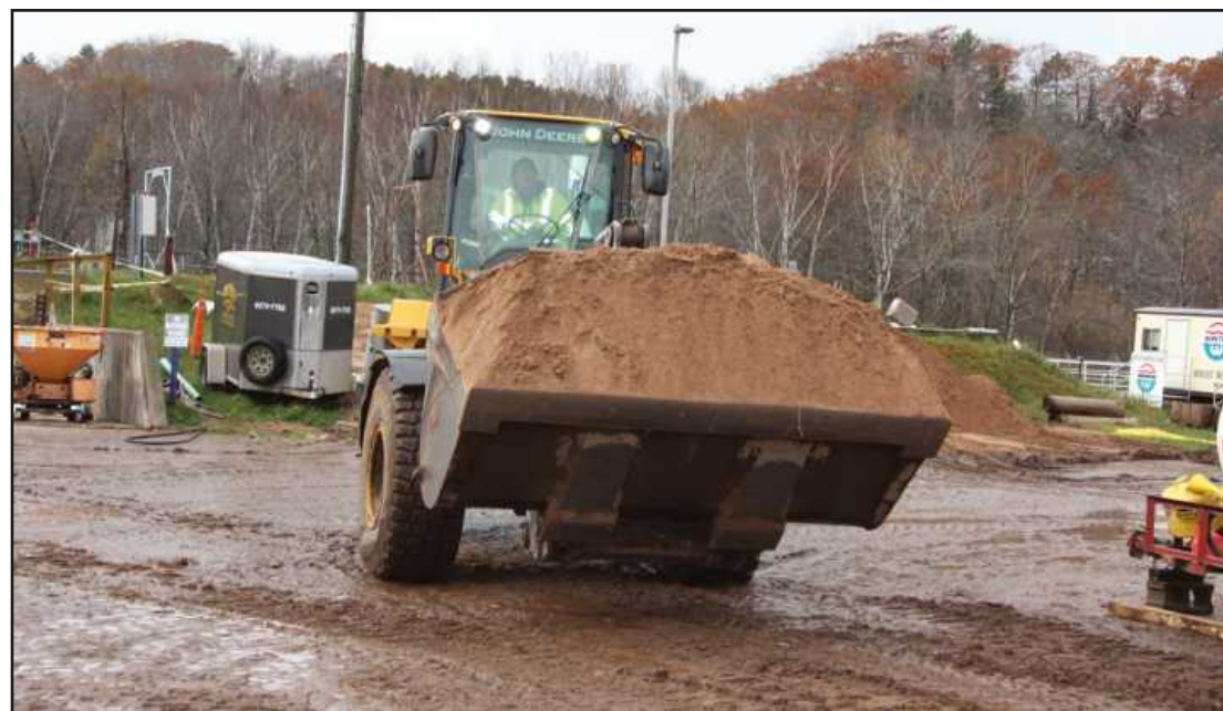
A LOAD OF DIRT IS ON THE MOVE at the Marquette Wastewater Treatment Plant project, and at the controls of the John Deere loader is David Rahoi of Operating Engineers Local 324. He's employed by M.J. VanDamme.
