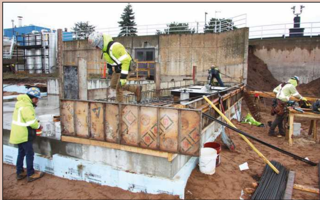
AT WORK CONSTRUCTING an addition to the Marquette Area Wastewater Treatment Plant are a group of iron workers and carpenters. They include Local 8 iron workers Nathan Petrovich and Brett Yuma (employed by SPE Inc.), and Local 1510 carpenters Jonas Christensen and Terry Lehtinen (employed by Miron Construction). Photo credits: Jack Deo
